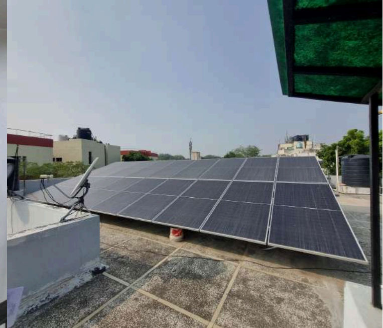
8kw Solar Project (Paschim Vihar)
