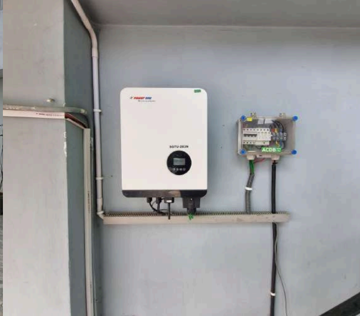
20kw Solar Project (District Center)
