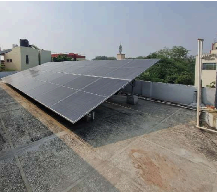
10kw Solar Project (Paschim Vihar)
