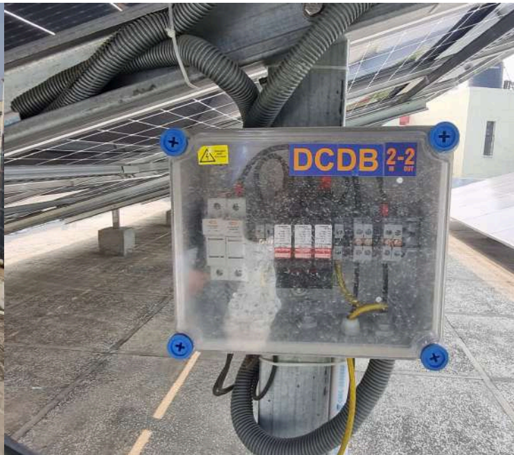
6kw Solar Project (Uttam Nagar)
